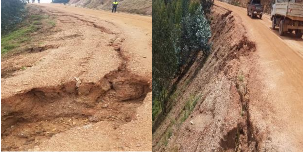
Photo taken by OAG on 6 th March 2020, showing erosion on road embankment
