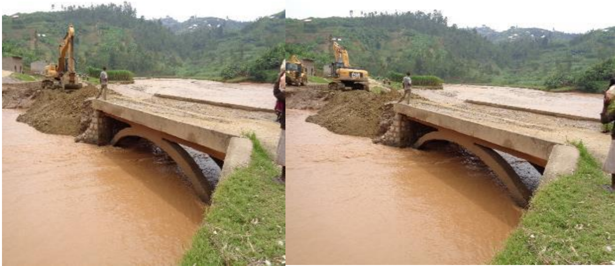
Photos taken by OAG on 4 March 2020: the spot 3 on Satinsyi River not yet constructed and bridge washed away by river.
