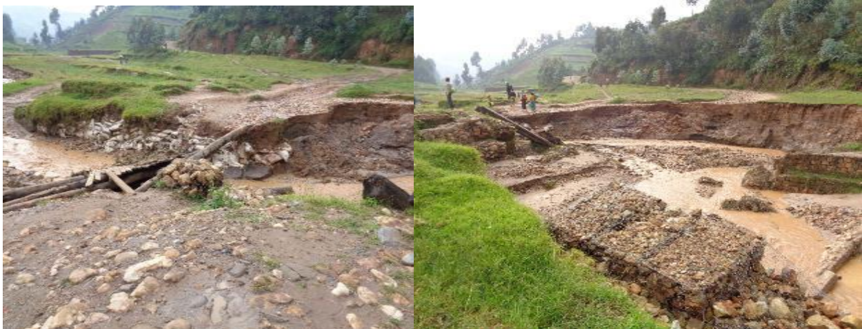
Photos taken by OAG on 4 march 2020: spot 5 not constructed and gabions washed out by rain (Rutsiro District/Gashyushya)
