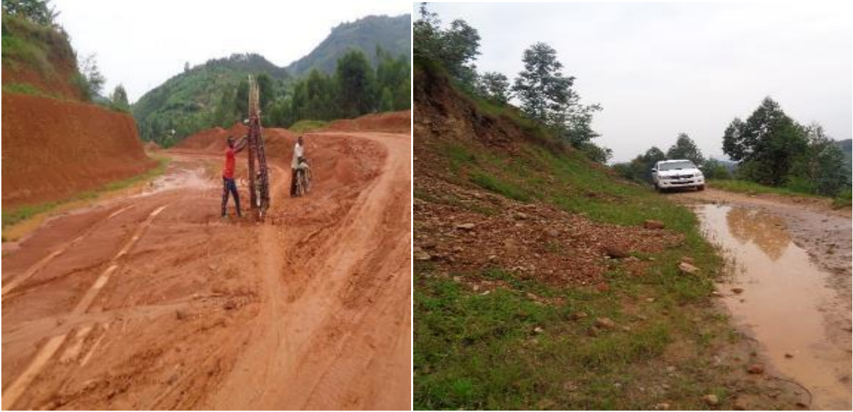
Example of sections where earthworks were ongoing and left uncompleted. (Photos Taken by OAG on 02 March 2020)
