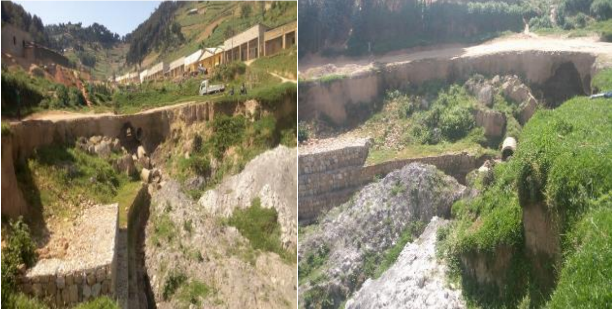
Photos taken by OAG on 4 March 2020: spot 6 not constructed and in bad condition (Rustiro District /Kavumu)
