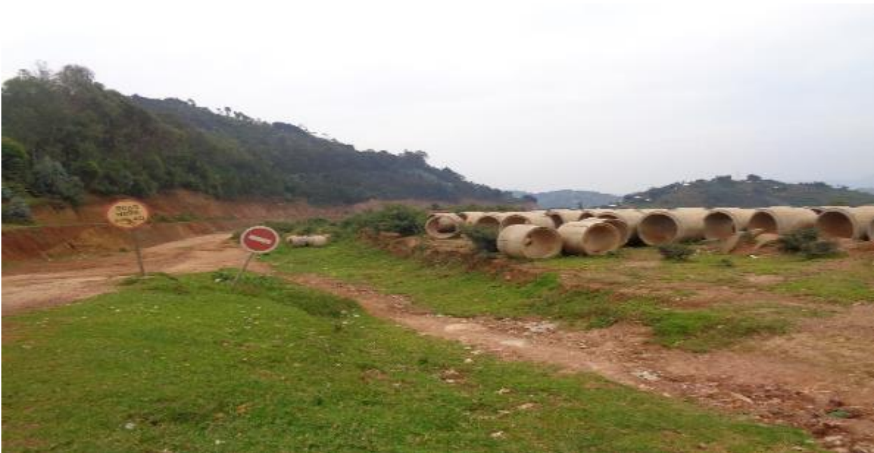
Section of the road which was closed due to unfinished earthworks. (Photo Taken by OAG on 02 March 2020).
