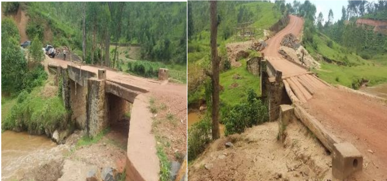
Photo taken by OAG on 6 th March 2020, showing Akanyaru Bridge not yet rehabilitated.
