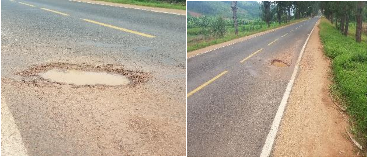
Photos taken by OAG on 6 th March 2020: Sections with potholes not yet repaired
