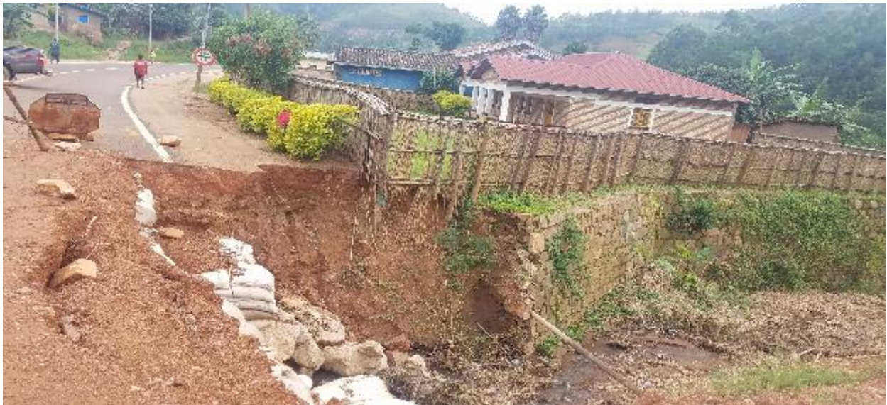
Photo taken by OAG on 6 th March 2020, showing a house in high risk
