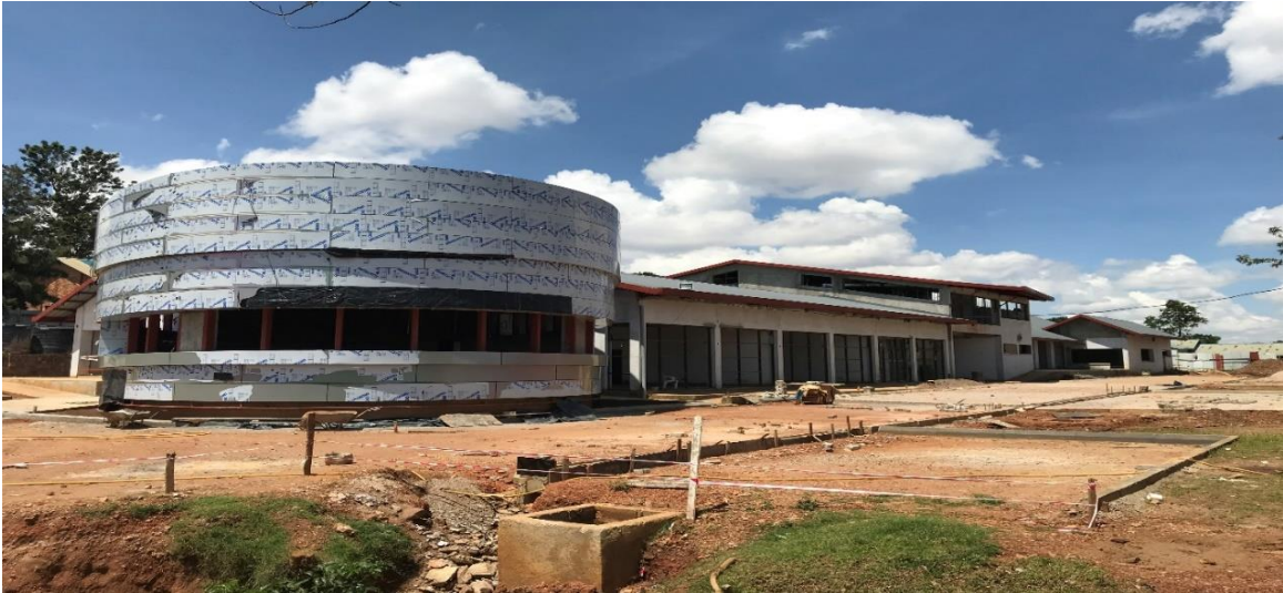
Incomplete works - front side of the building: Photo taken by OAG on 18 March 2020
