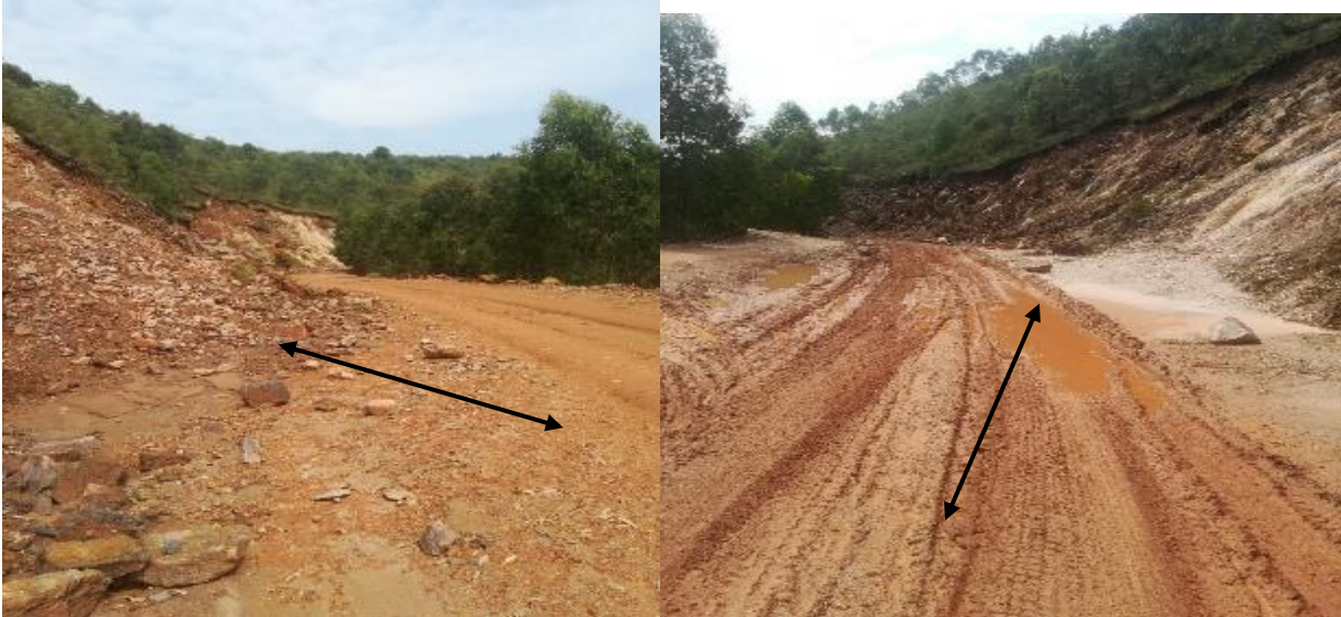
Photos taken by OAG on 3 March 2020: the landslide fall down on the road and damaged carriage way.
