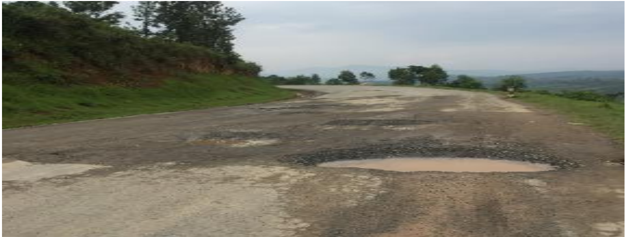
Photos taken by OAG on 6 March 2020: The section of the road seriously damaged
